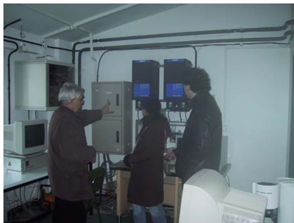
PV control and monitoring system
