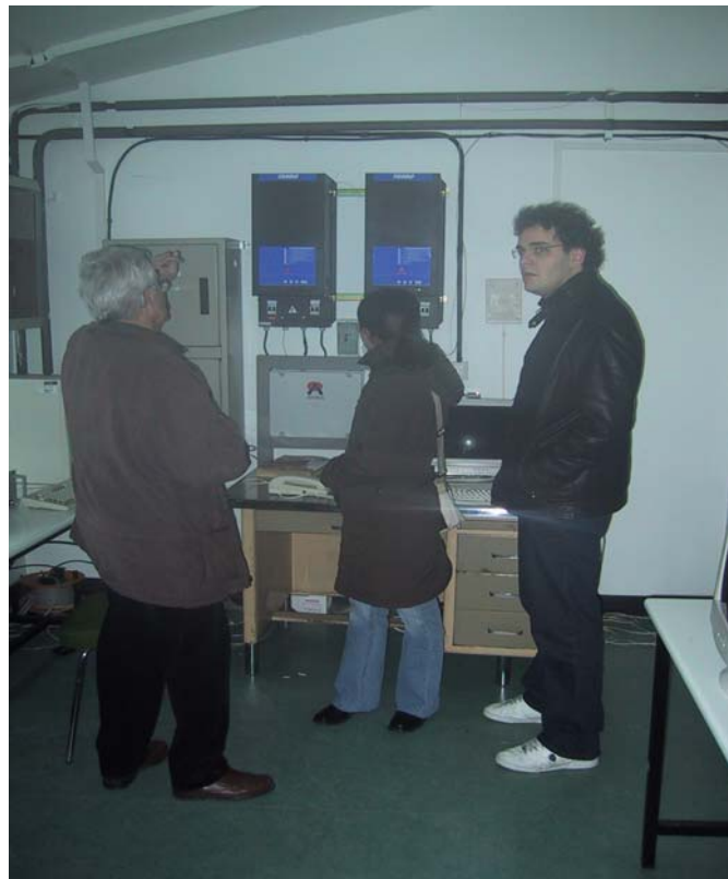
PV inverter system
